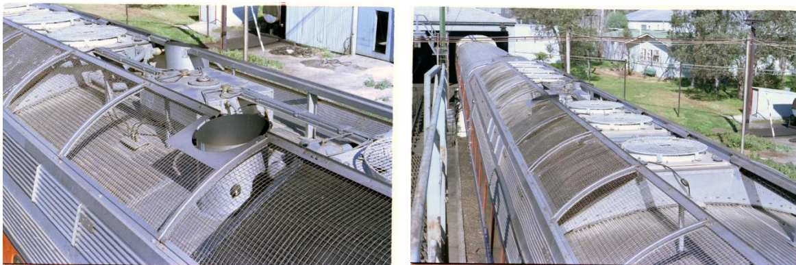
Details of roof, radiator fans and exhausts
